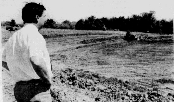
Construction is underway on two catfish ponds as part of a research project.
