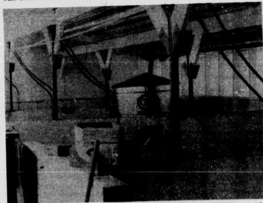
The Swine Feeding Floor (above) looks almost ready for its residents to move in as work on it moves into the final stages with only the hanging of lights and a little painting to be done.
