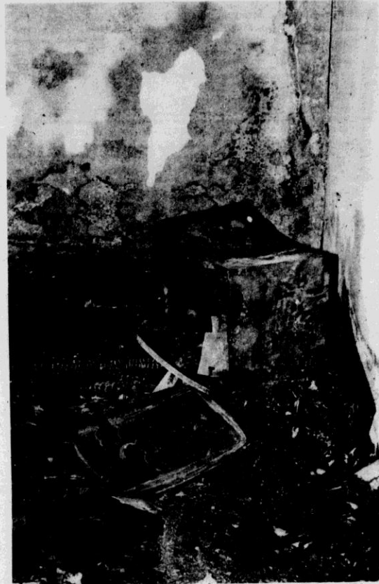
ABOUT THE only real casualty from the Lucas Hall fire Tuesday morning was the basement lobby television. The TV, along with all the lobby furniture, the pay phone and light fixtures, was completely destroyed in the blaze which spread smoke and soot throughout the dorm and caused a large amount of plaster to fall off the lobby walls.
